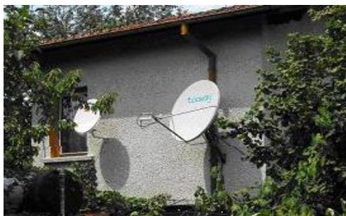
Antenna and ODU installed on a wall
